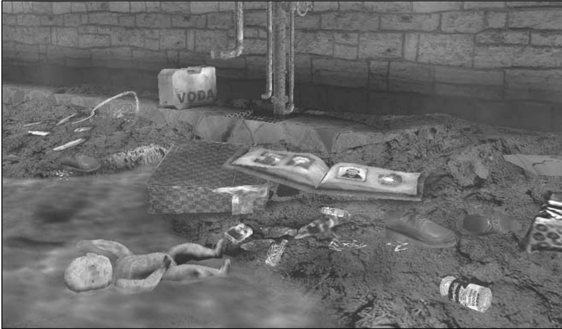
Figure 1: Objects in the culvert.
